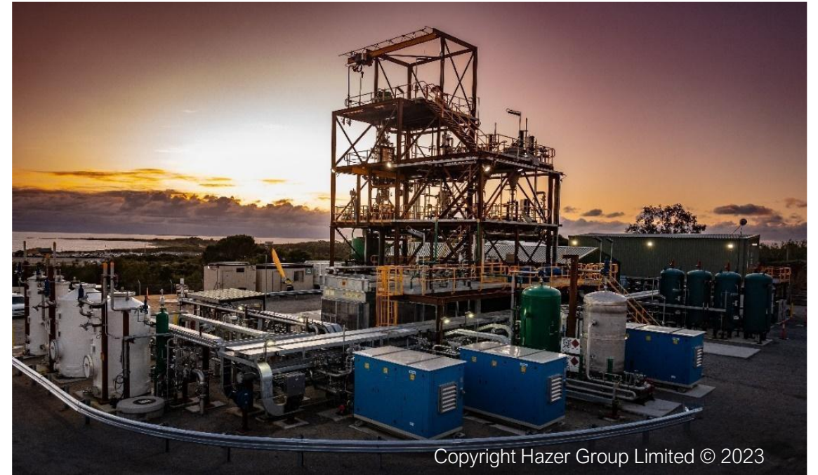
Hazer Group commercial demonstration plant Perth, Australia
